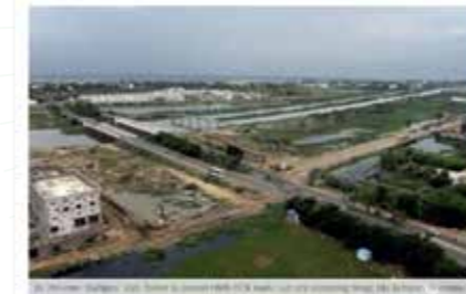
The Chennai Metro Rail Limited (CMRL) has decided to construct a road-like flyover to connect OMR-ECR roads in the style of Kattipara in Chennai.
