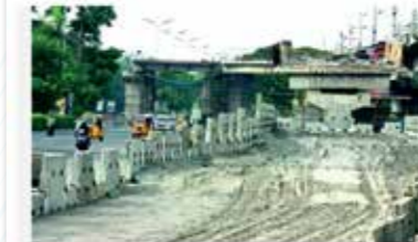
Chennai Of the two U-shaped flyovers being constructed at 106 crore on Old Mahabalipuram Road (OMR) in Taramani, the one near Indira Nagar junction is likely to be opened for public use within the next two months.
