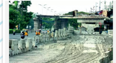
Chennai: One of the two U-shaped flyovers being constructed at MB entrance on Old Mahalingapuram Road (OMR) in Taramani, the one near Indira Nagar junction is likely to be opened for public use within the next few months.
