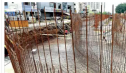
The metro drains are to restore the original stream routes
